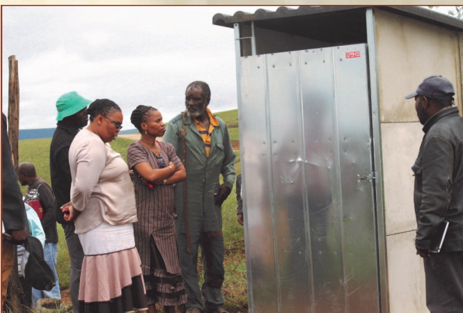
Executive Mayor, Mayor of Mbizana Cllr. Twabu and Cllr. Busuku Checking VIP Toilet at Lucwaba Village in Mbizana during
